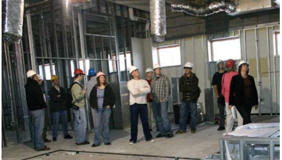
Alliance Construction Solutions provided Construction Management and CAD/Engineering students an up front view of the renovations at Ed Beaty Hall. (See more pictures on Page 4.)
